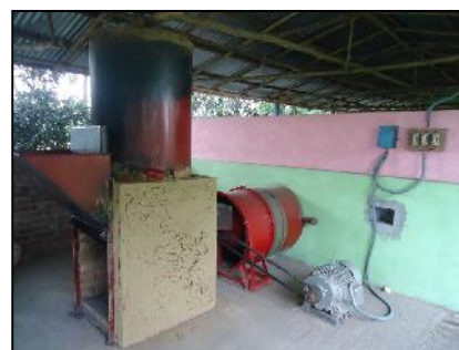
Figure 2: Conventional Flatbed Dryer – Jessore pilot
