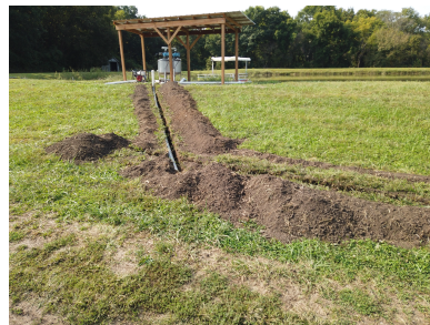
Water line from holding pond to plots.
