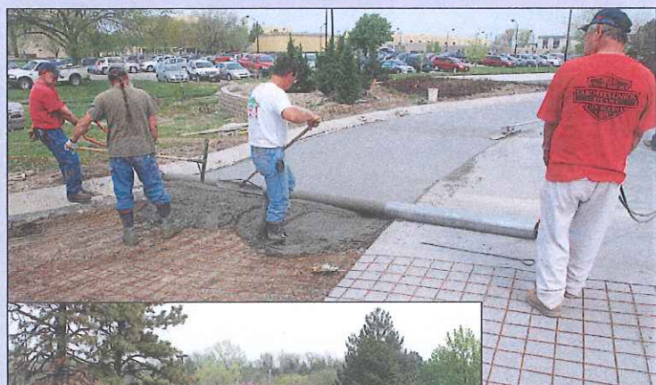
Pouring concrete for the new drive (top); at left, new blocks for materials storage have been installed.
