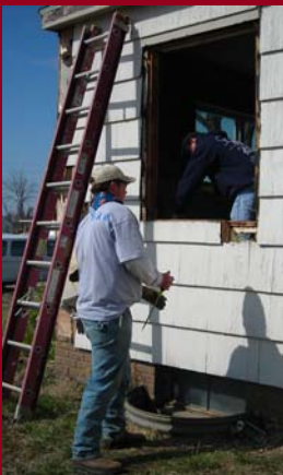
Daniel Stanford and Adam Marcotte of Pratt Community College help rebuild a Chapman, KS house (photo courtesy of Kansas Corps)
